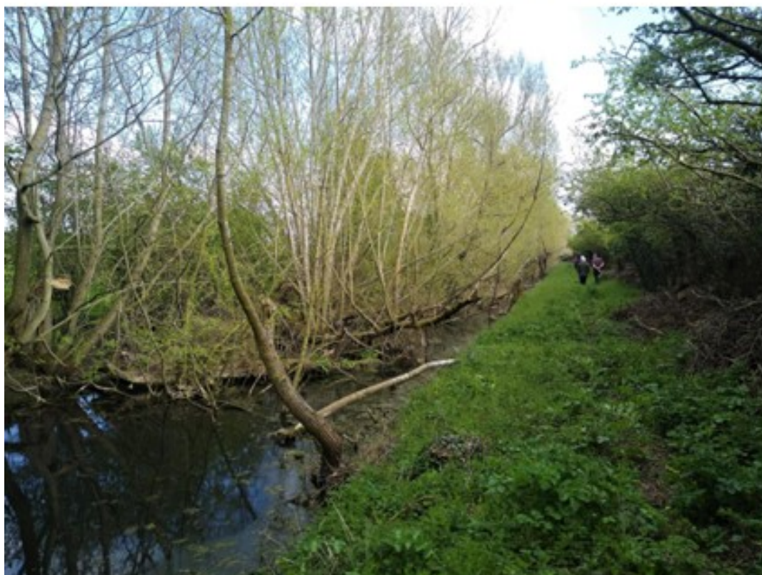
Current view of the canal between Crews Pitch and Skew Bridge; now completely clogged with fallen timber. Work is needed urgently to save these old Pollard Willows and to restore clear water for the benefit of the wildlife species which require open water.
