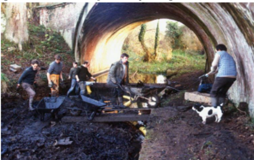
Restoration work at Skew Bridge in the 1980s with volunteers from the Waterways Recovery Group.
