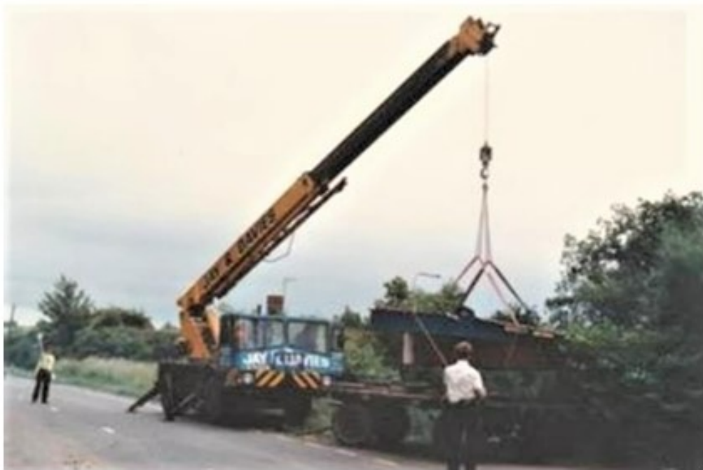
1995 – Unloading a boat and craning it in to the canal from the main road
